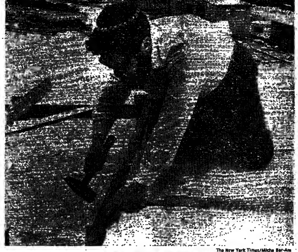
Yosef Porat, a volunteer from the Kiryat Arba settlement, works on the roof of a new dining room at Camp Kadum. Newly installed bouse trailers are in the background.
